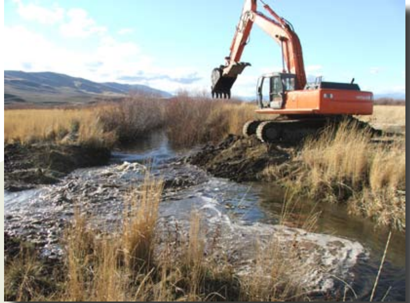
With the grade control structures in place, a backhoe operator breaches a temporary de-watering dam, allowing water from Mid-Toppenish Creek to flow along its historic channel. (Photo courtesy Tracy Hames.)
